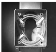
Presets have room to store up to 1 meter of cable in preset. Fiber loop clips (Cat. No. 427) shown.
