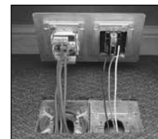
Flush activations offer a full range of power and communication connections.
